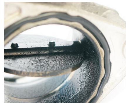
Regulating throttle suffering from oil contamination
